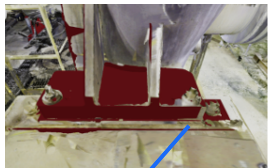
Baseplate fit-up issues required field and shop machining
